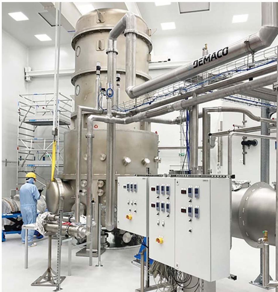
Figure 4. Mirror tower in the ETPATHFINDER facility. The tower has a height of 6.1 m and a diameter of 2.8 m. Credit: ETPF Project [2]
