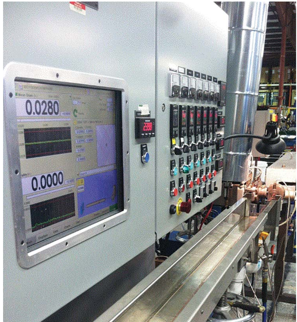
Extruder view shows the extrusion line panel at the Pelican Wire facility in Naples, Florida. Credit: Pelican Wire
