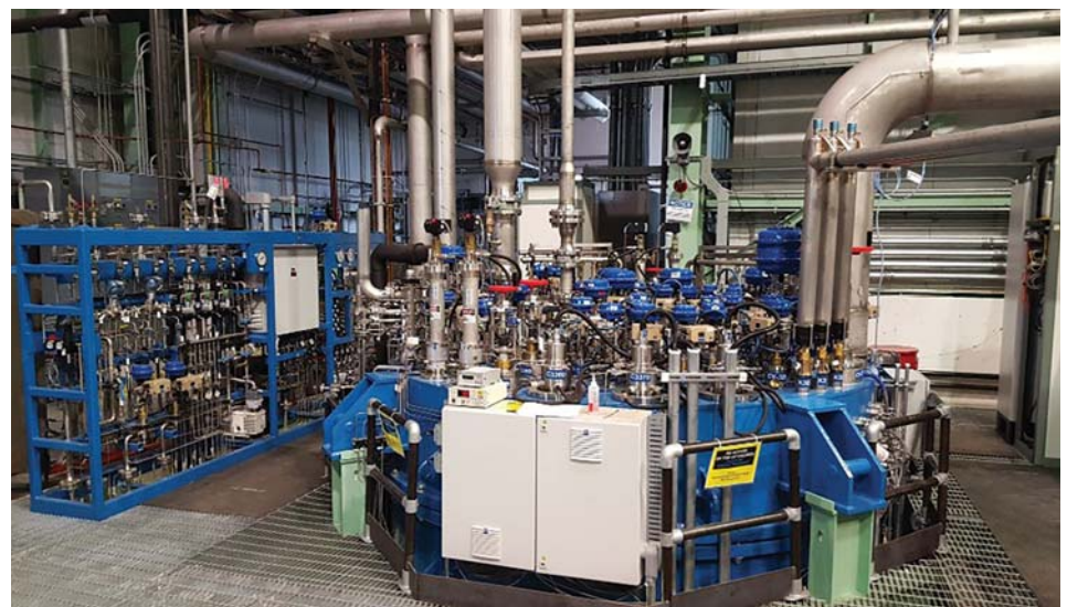
Figure 3: Industrial cryoplant at Fermilab's Cryomodule Test Facility. Credit: FNAL
