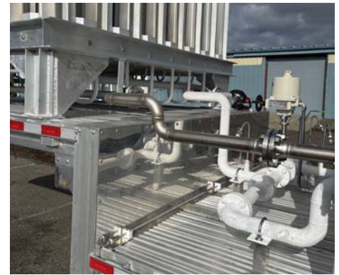
Piping undergoing cold shock testing. Credit: Spaceline Technologies
