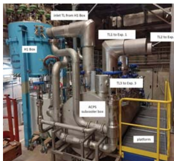
The ALPS cryoplatform subcooler box (ACPS) in the hall HERA North. Credit: DESY
