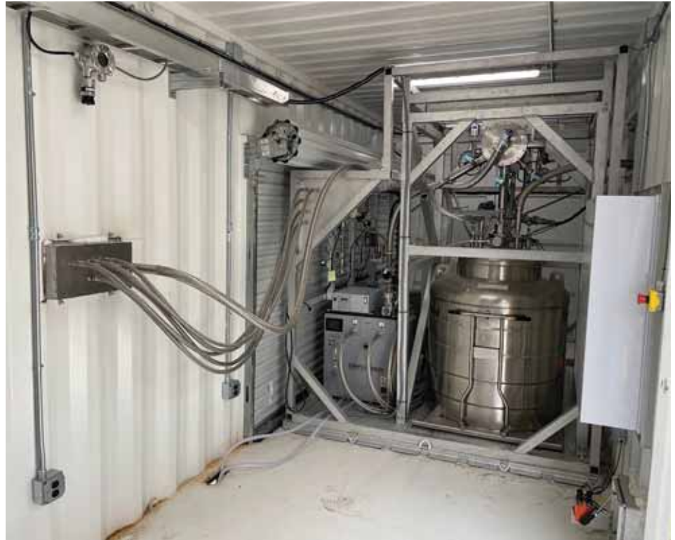
Hydrogen liquefaction and controlled storage system LS20 for small-batch LH 2 supply. Credit: GenH 2 (J. Fesmire)
