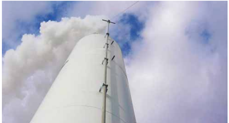
Typical bulk storage tank venting GH 2 to relieve pressure. Hydrogen venting losses can exceed 20%, with actual 'real-world' losses at or near 40%. Credit: GenH2
