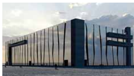
Construction is getting underway at the IFMIF-DONES site in Granada, Spain. Credit: IFMIF-DONES
