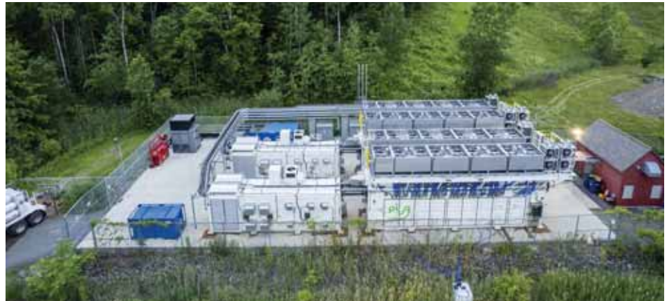
Microsoft's 3-MW hydrogen electric cell system in Latham NY, includes two 40-foot containers, each holding 18 proton exchange membrane (PEM) cells by Plug. A gaseous hydrogen tube trailer is seen at left. Credit: John Brecher, microsoft.com [3]
