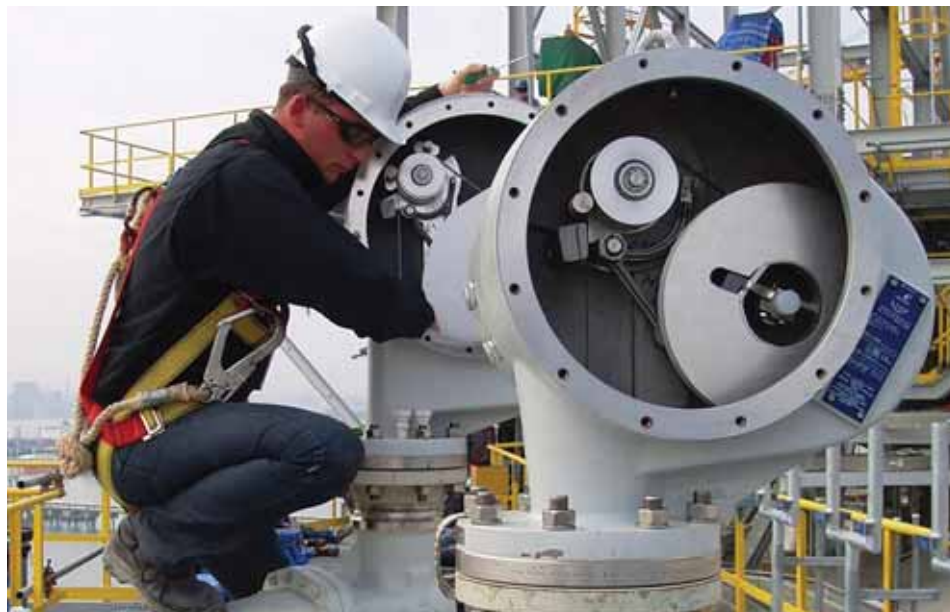
Svanehøj and Engie are teaming up to enhance offshore LNG safety on FSRUs. Svanehøj's advanced technologies monitor and control LNG storage conditions, while Engie Lab Crigen conducts simulations to analyze offshore storage risks. Credit: Svanehøj
