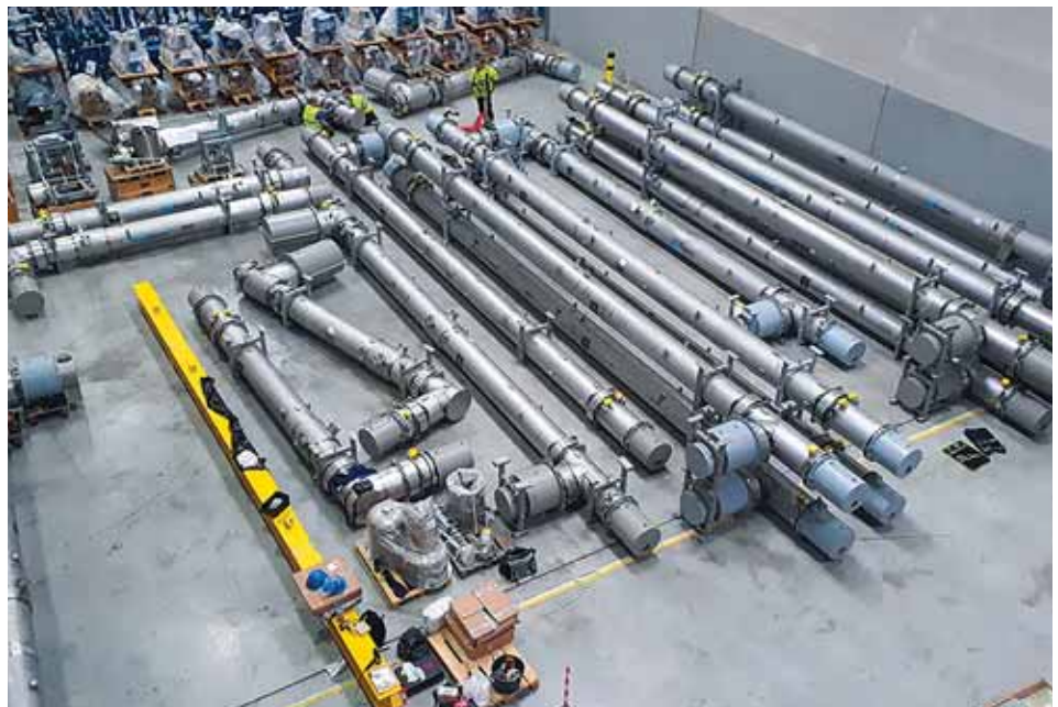
Cryo connections: Cryogenic bypass lines supplied to FAIR through an in-kind contribution by WUST in Poland. Credit: GSI
