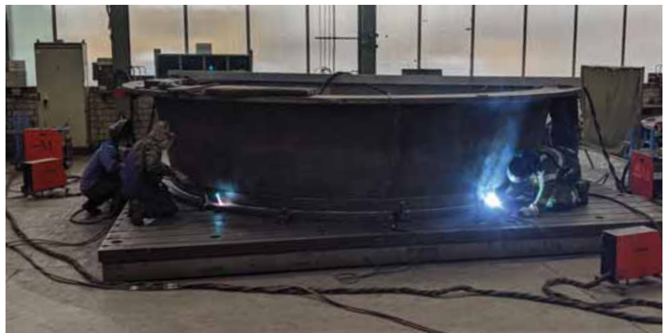
Welding of the FYST support cone base assembly. Credit: CCAT Observatory, Inc.
