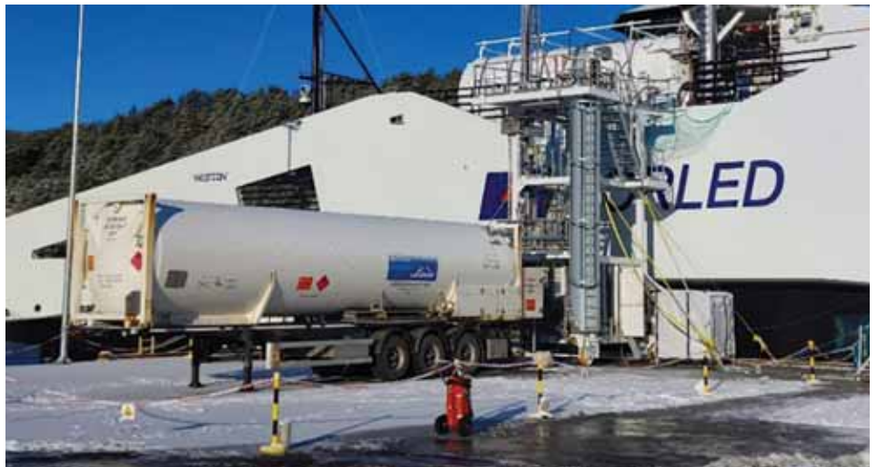
Figure 2. Bunkering station with the LH 2 tanker trailer connected to the onboard LH 2 storage tank. Credit: Linde
