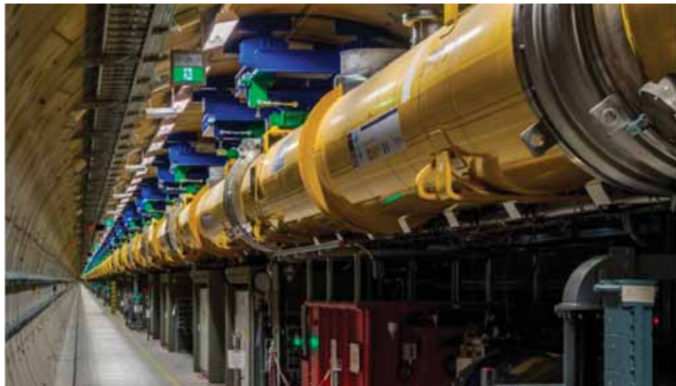
Figure 5. SRF accelerator in tunnel of European XFEL. [10] Credit: Reschke et al.
